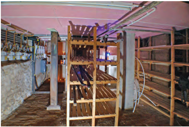
View of the roomy cellars below number 16-18. The far wall is given over to storage bays
